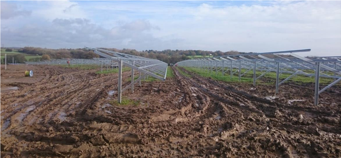
Inserts 36 and 37: Winter Installation (2015) and Operational Site (2022)
